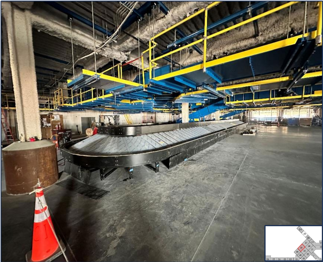
Installation of Outbound BHS Carousel in Zone 28 of the Main Terminal
